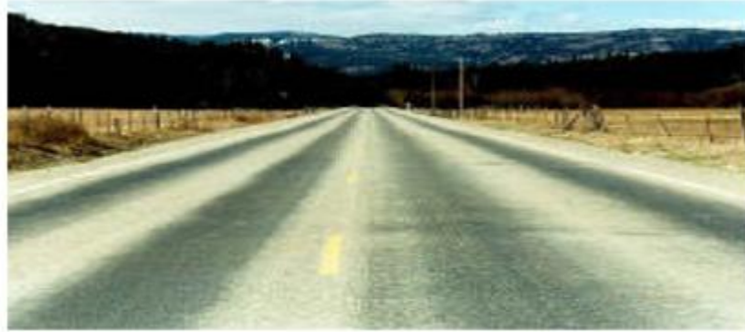
Figure 22 Bituminous Surface Treatment Bleeding in Wheel Paths
