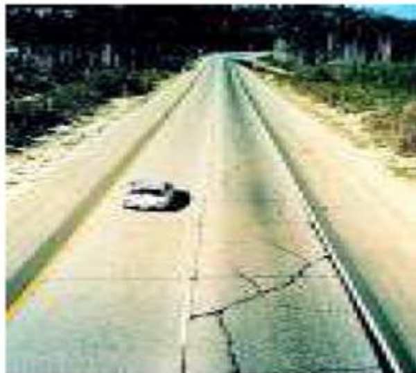
Figure 75 Panel Cracking in the Truck Lane
