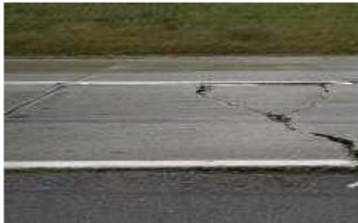
Figure 73 Large Panel Crack
