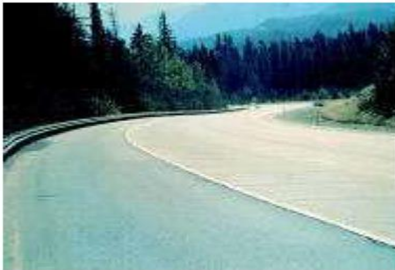
Figure 70 Faulting in the Truck Lane
