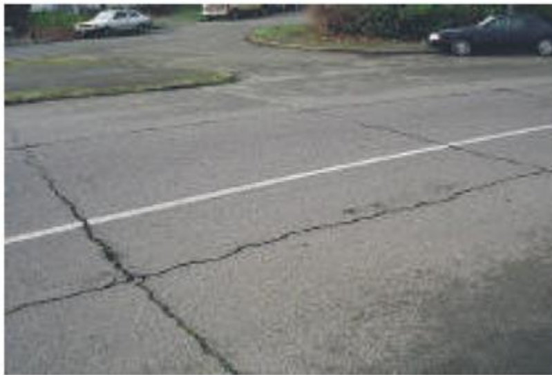
Figure 27 Joint Reflection Cracking on an Arterial
