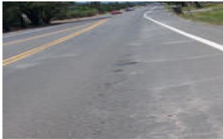
Figure 48 Cement Treated Base Pumping through HMA Cracks
