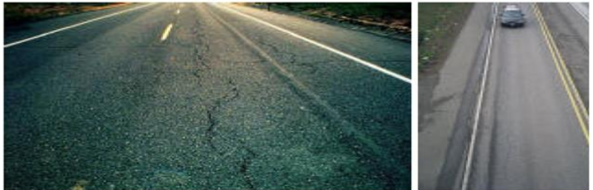
Figure 29 Longitudinal Cracking as the Onset of Fatigue Cracking
