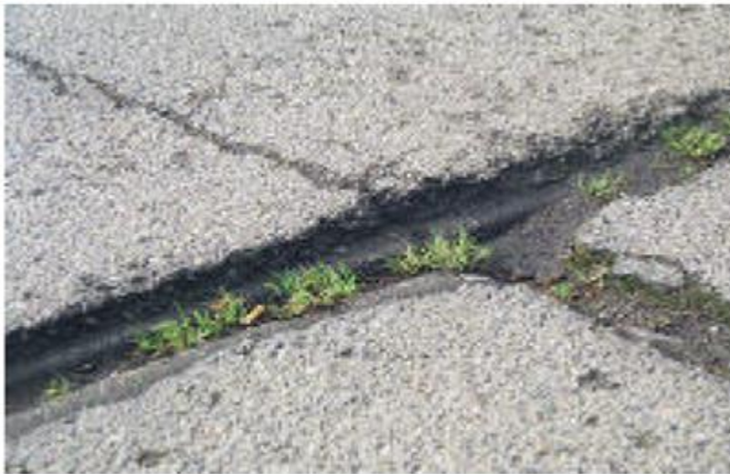
Figure 28 Joint Reflection Cracking Close-Up
