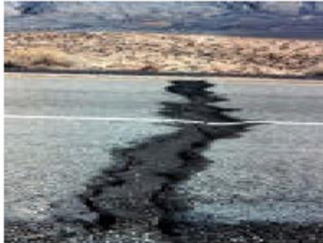
Figure 44 Large Patched Thermal Crack
