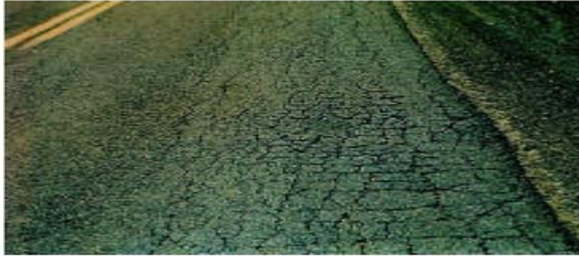
Figure 19 Bad Fatigue Cracking
