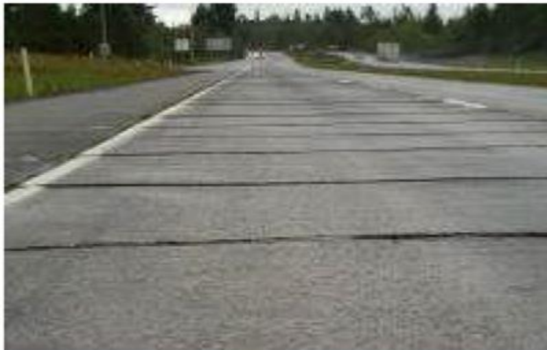
Figure 69 Faulting from Ground Level
