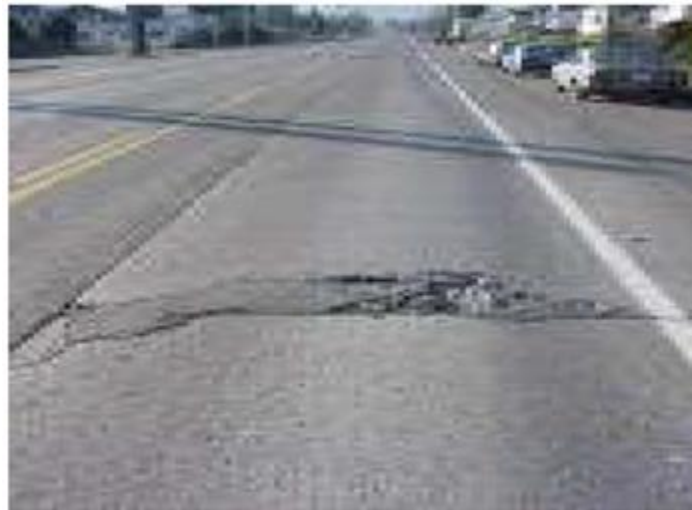
Figure 91 Spalling from a Bad Construction Joint
