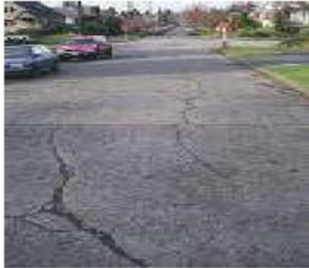
Figure 74 Panel Crack on a Residential Street
