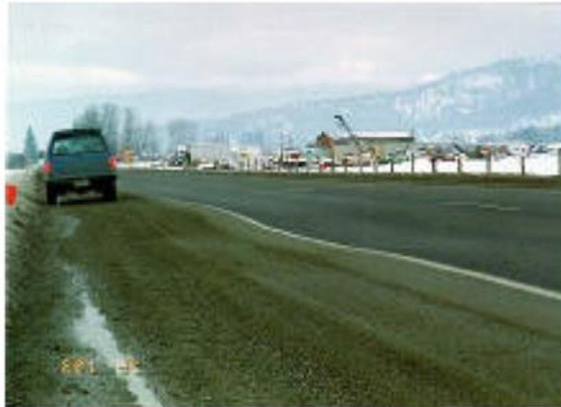
Figure 26 Depression in Left Lane and Shoulder
