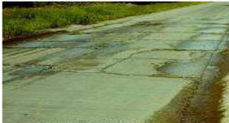
Figure 84 Broken Slabs with Pumping Evidence
