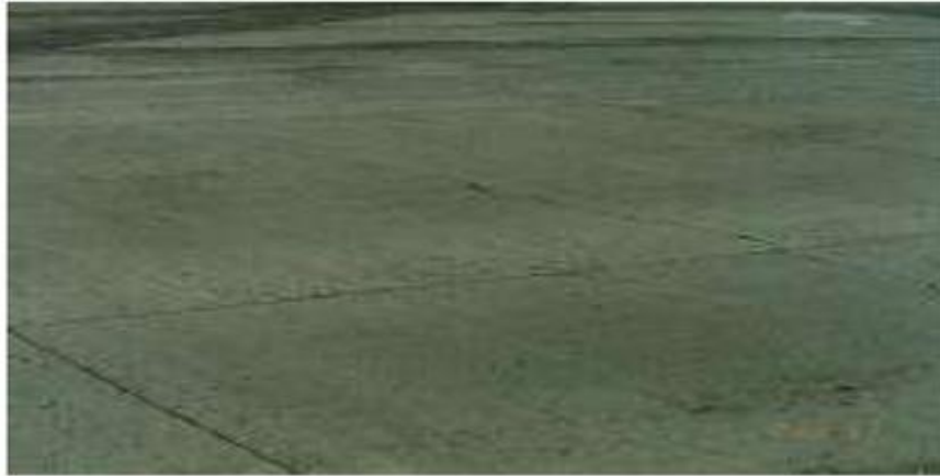
Figure 88 Shrinkage Cracks on Brand New Slabs
