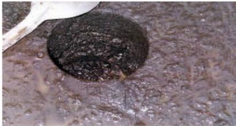
Figure 41 Core Hole showing Stripping at the Bottom
