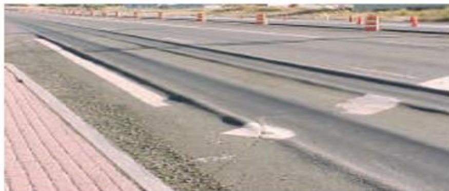
Figure 39 Rutting from Mix Instability
