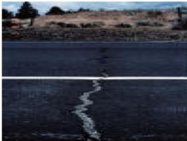
Figure 45 Smaller Patched Thermal Crack
