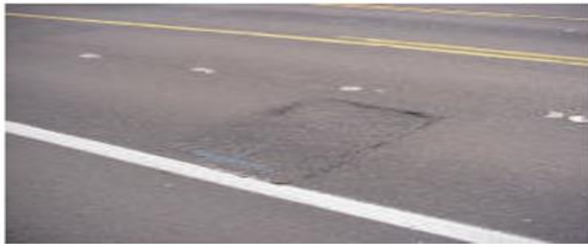
Figure 32 Patch over Localized Distress
