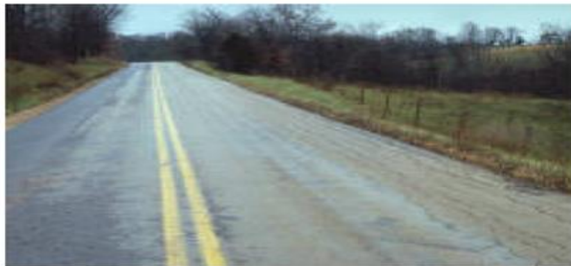
Figure 21 Fatigue Cracking from Edge Failure
