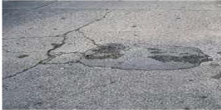
Figure 76 Patching on a Residential Street
