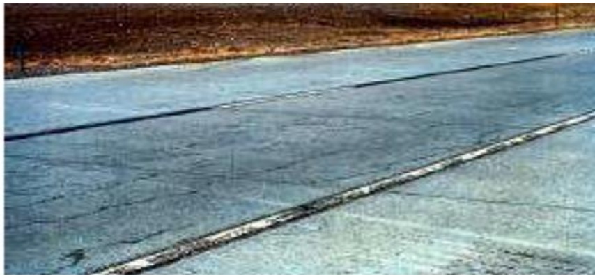
Figure 89 Severe Shrinkage Cracking
