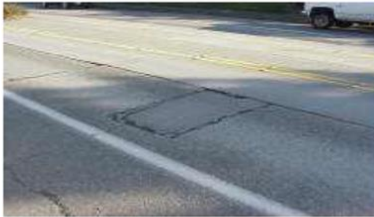
Figure 77 Patching with Poor Edges
