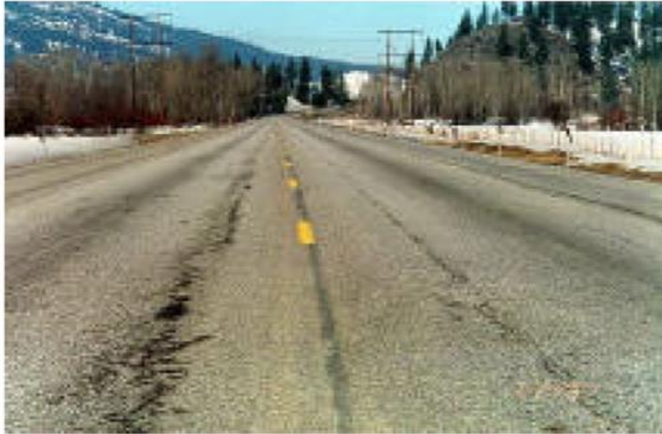
Figure 49 Raveling Due to Low Density
