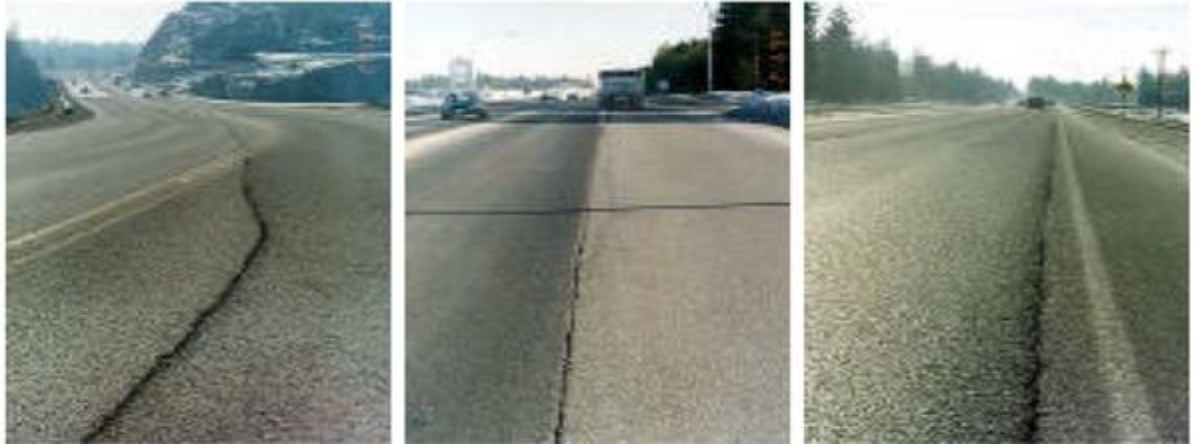
Figure 30 Longitudinal Cracking from Poor Joint Construction
