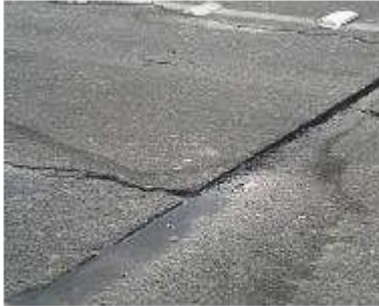
Figure 71 Faulting Up-Close a Bus Stop
