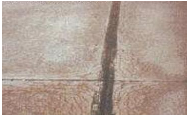
Figure 68 D Cracking at Panel Corners
