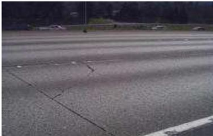
Figure 67 Corner Break on a Highway
