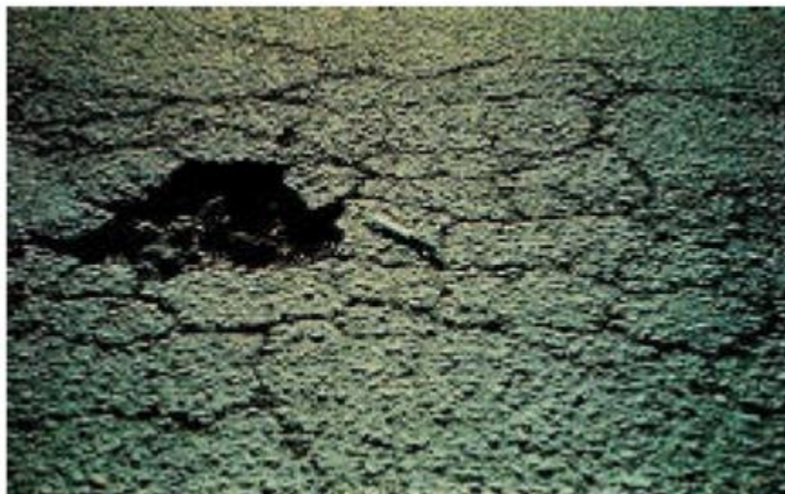
Figure 36 Pothole from Fatigue Cracking
